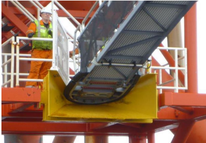
Figure 26: V-shaped landing zone for the motion compensated gangway, [source: [76] with permission by Ampelmann].
