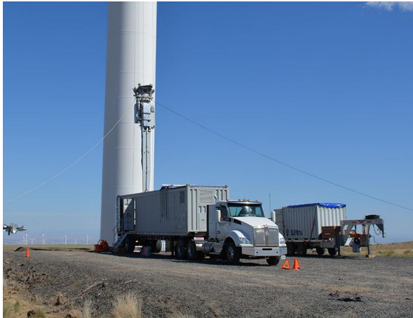
Figure 40: Self-hoisting crane climbing its own lifting wire from its container to the nacelle, [source: [107]].
