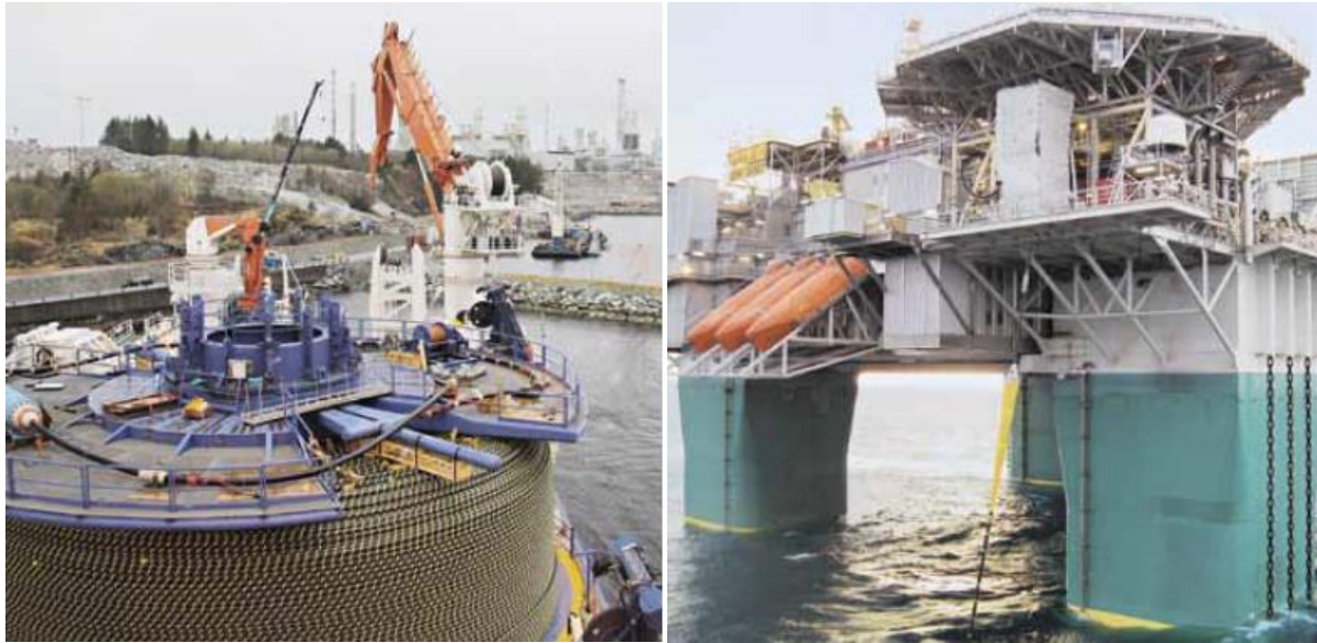
Figure 5.1-11 – Left: Cable drum on CLV at cable landing location; Right: Cable being pulled with messenger wire onto platform (yellow = bend stiffeners); Source: [16]
